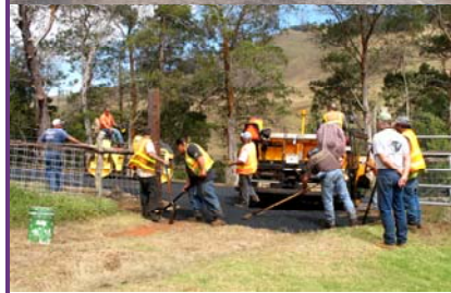
Clarence Tavares [top photo on right] and Sonny Vic Paving crew pave road and entrance gate to Pu'u Mahoe.
